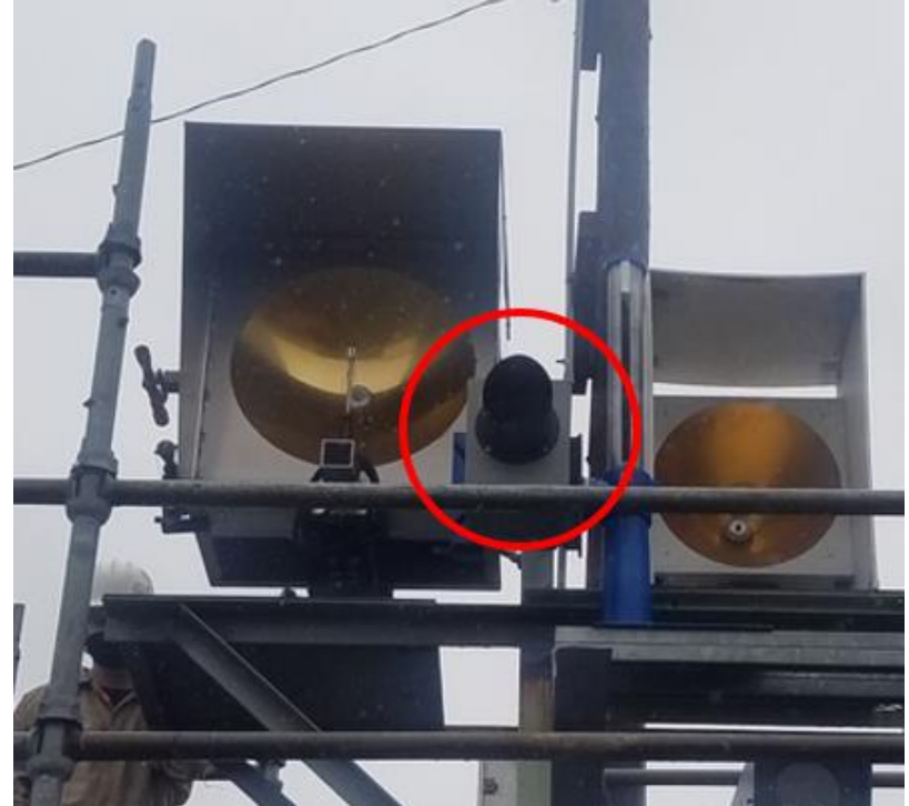
Retroreflector Mounted on the Reflector Tower
