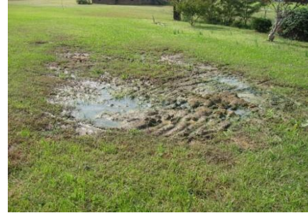
Septic system failure
