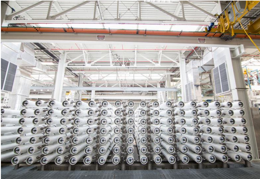
Orange County Water District (OCWD) Groundwater Replenishment System (GWRS) Reverse Osmosis (RO) Facility
