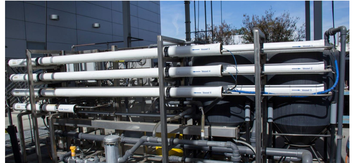
Orange County Water District (OCWD) RO pilot test system
